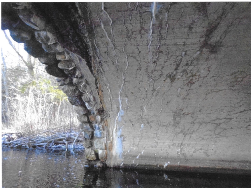
Photo 6: Typical map cracking and heavy efflorescence 5' into concrete section with evidence of wetness and moderate scaling at arch interfaces (northeast corner shown)
